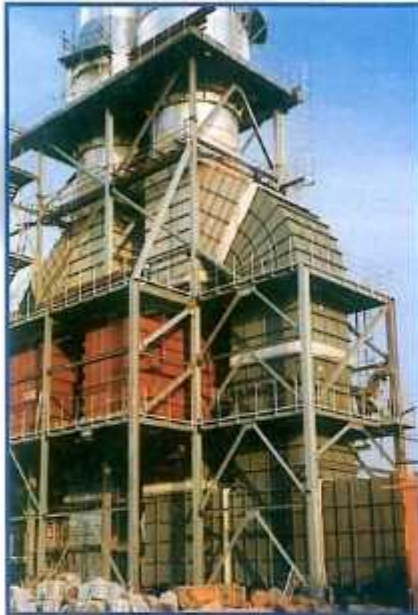
Gas turbine plant with DEKOMTE Flexible Expansion Joint
